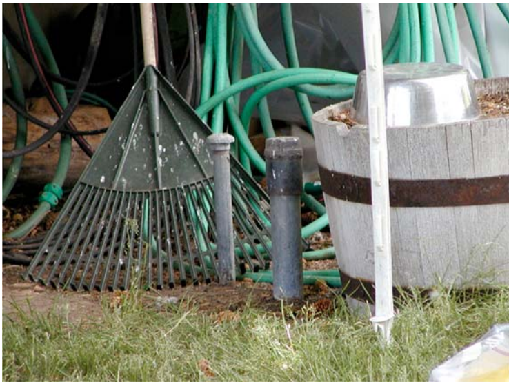
FIG. X1.7 Fill pipe and vent pipe leading to an underground storage tank containing fuel oil in the yard of a single family home.
